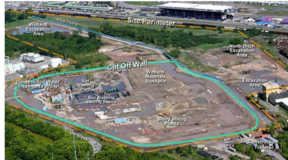
Figure 1: An aerial photo of the LCP site when surface soils were being processed to remove mercury. The Grandstand at the NYS Fairgrounds can be seen in the background. The turquoise line shows the approximate placement of the slurry wall which is designed to prevent contaminants from leaking off-site. The wall consists of a trench dug 30-70 ft into the earth, filled with bentonite clay.
